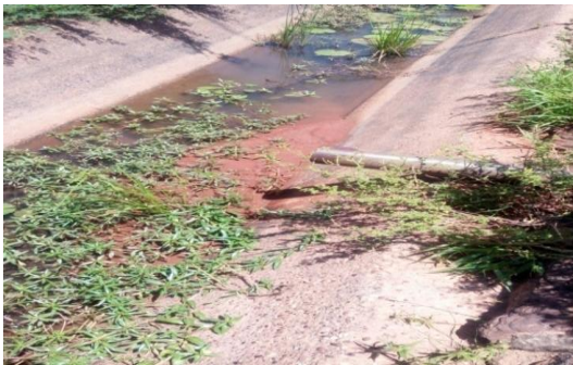
Figure 4: Seepage flow containing eroded material from the dam
