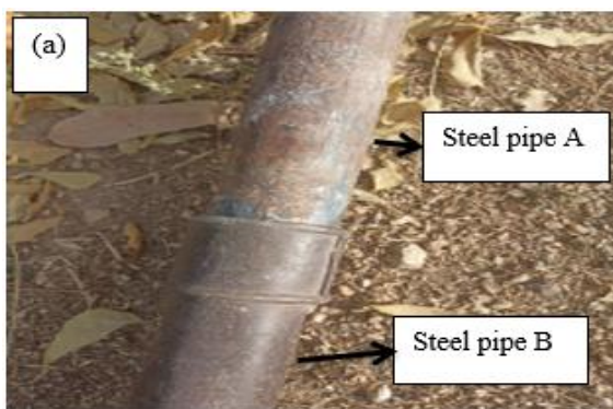
Fig. 1: Steel pipes from a borehole site (a) Couple steel pipes removed from a borehole
