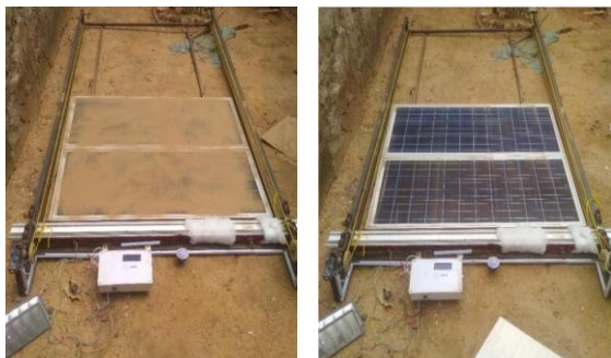
(a) System with Dust (b) System after cleaning
